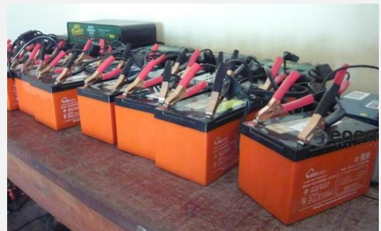
Figure 12 : Batteries used for the battery swap in Tanzania by EGG-Energy, a social business sponsored by ENEA Consulting.
