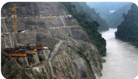
The Subansiri dam project in India (Source: The Hindu / Ritu Raj Konwar)
