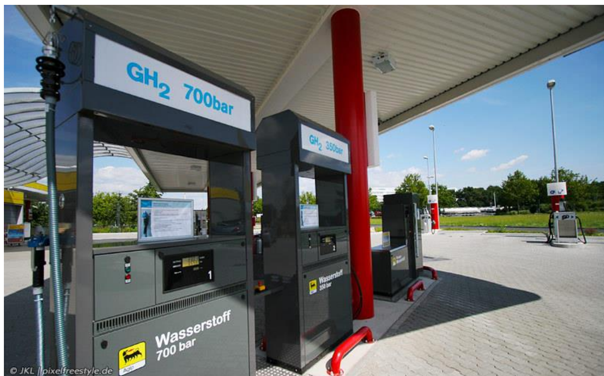
Figure 8: A hydrogen refuelling station in Frankfurt-Höchst
